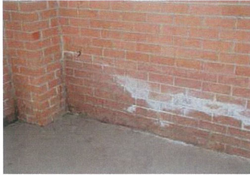
Figure 4: Efflorescence; the result of soluble salts that migrated to the surface (Source: Think Brick Australia, Industry Reference Guide, Fifth Edition 2009)
