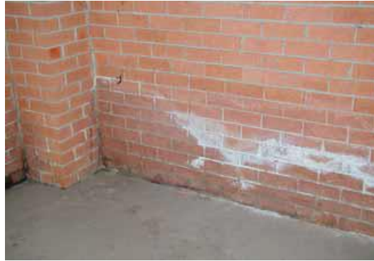
Figure 4: Efflorescence; the result of soluble salts that migrated to the surface (Source: Think Brick Australia, Industry Reference Guide, Fifth Edition 2009)
