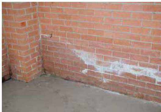
Figure 5: Efflorescence; the result of soluble salts that migrated to the surface (Source: Think Brick Australia, Industry Reference Guide, Fifth Edition 2009)
